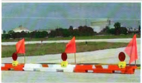
VEHICLES AND LIGHTS THAT MEETS THE MOST CURRENT VERSION OF THE FAA AC 150/5320-200 TO PLACE AND MAINTAIN RED SOLAR BARRICADE LIGHTS FOR RUNWAY END (I.E. FILLED WITH WATER) TO AVOID BEING MOVED BY JET BLAST SET 4' END TO END MINIMUM OR AS DIRECTED BY THE ENGINEER. THE LIGHTS SHALL BE MARKED WITH THE CONTRACTOR'S NAME OR LOGO, DIAGONAL, ALTERNATING ORANGE AND WHITE STRIPES.
